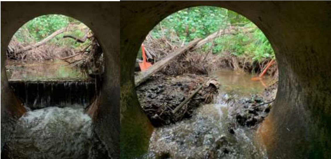
Figure 6: Fish barrier remediated in a tributary of the Waikawa Stream. Photo on the left shows prior to remediation (a drop due to a wooden board covering entrance to culvert) and photo on the right after remediation by removing the board.
